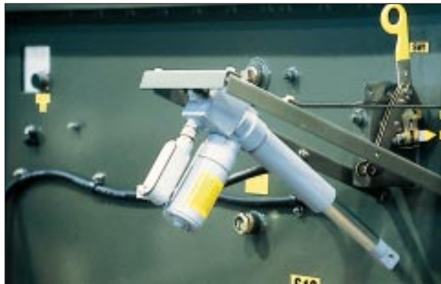
DC Motor Actuator - Disconnected.
